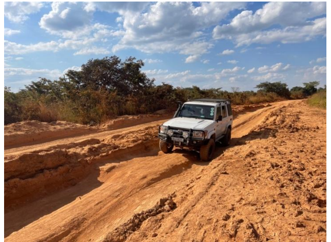
Chainage 86 +000 – Section in poor condition
