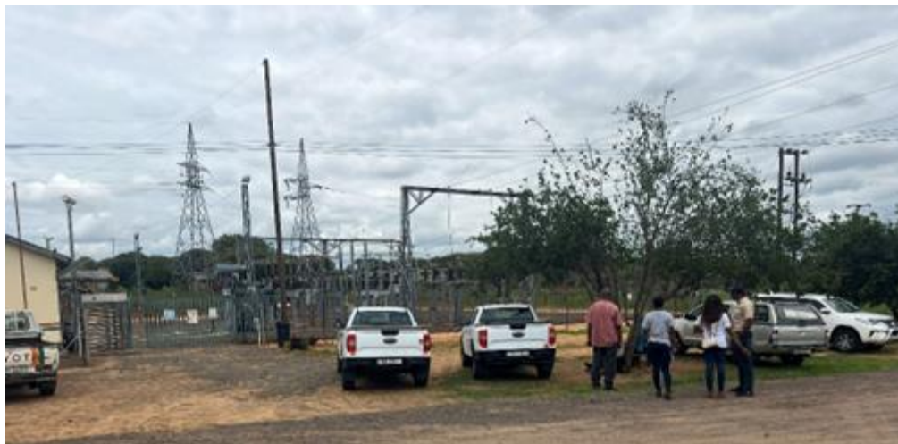
Visit to Kazungula ZESCO substation
