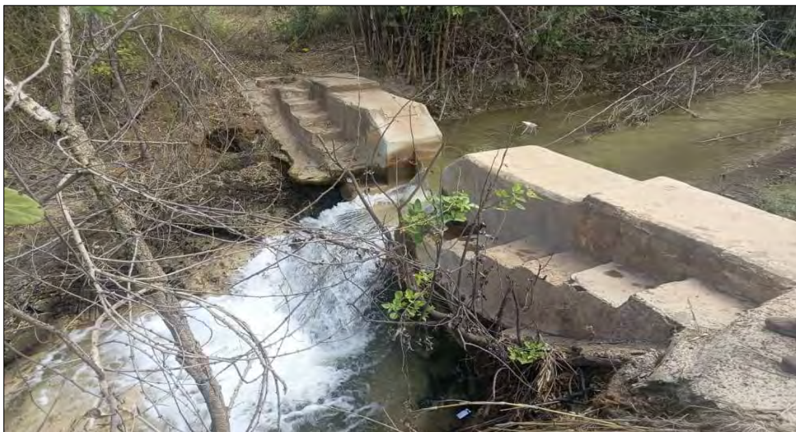
Figure 4-76: Photograph showing v-notch weir at the discharge from New Dam to Chambishi Stream
