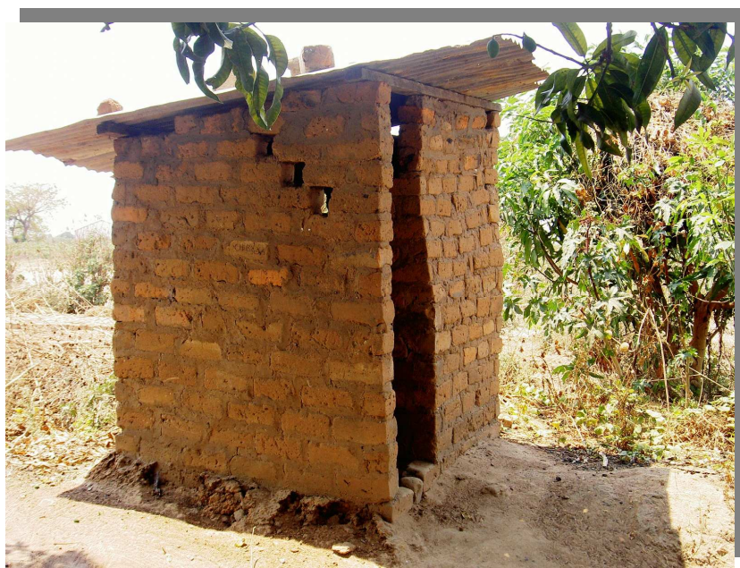
A toilet in a peri-urban area (NWASCO, 2006)
